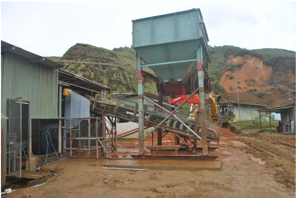
Testing and modifications are continuing on the newly installed mechanical ball mill feeding plant
